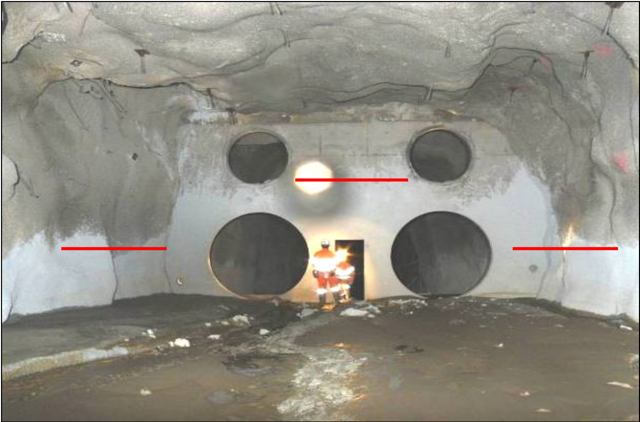
Photograph 3: Ventilation wall about 350 m from the base of VR5A shaft. The two outer red lines show the approximate height of the inrush flow. The centre red line shows the height of the turbulent flow when it splashed on the ventilation wall.
