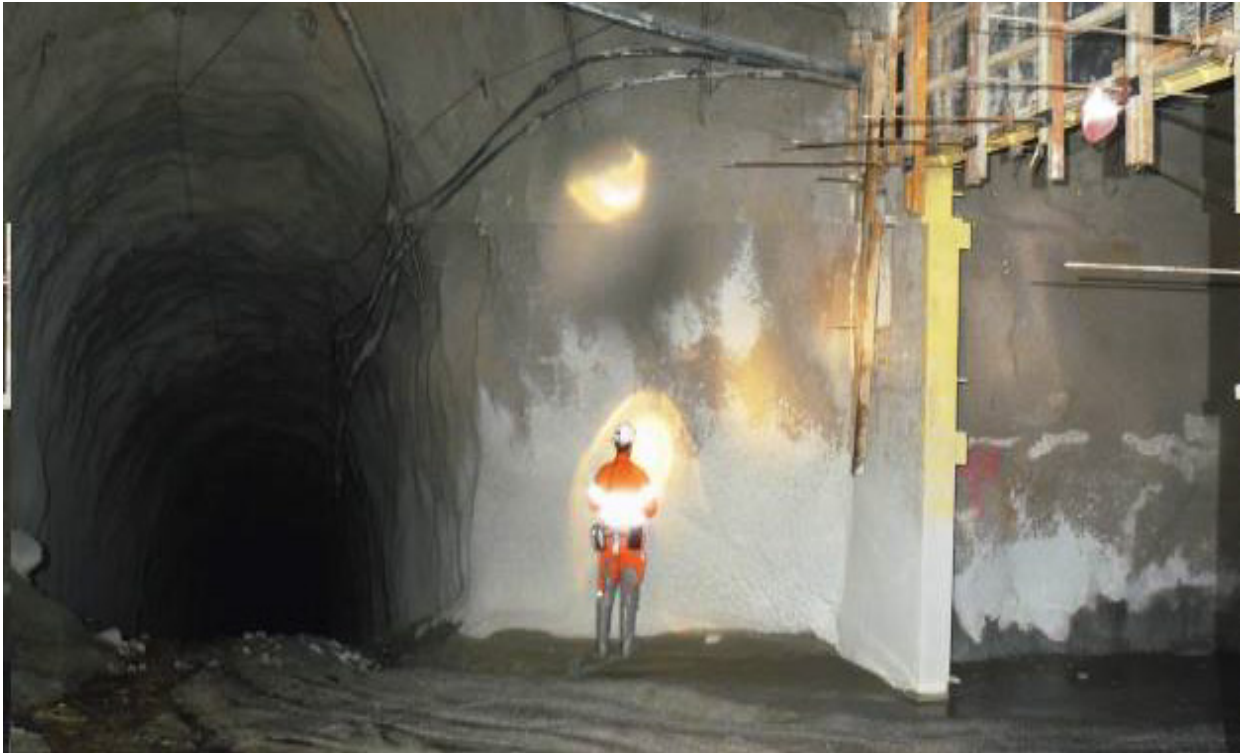
Photograph 4: The roadway intersection 550 m from base of VR5A shaft showing the height of the turbulent flow on the wall beyond the ventilation structure.
