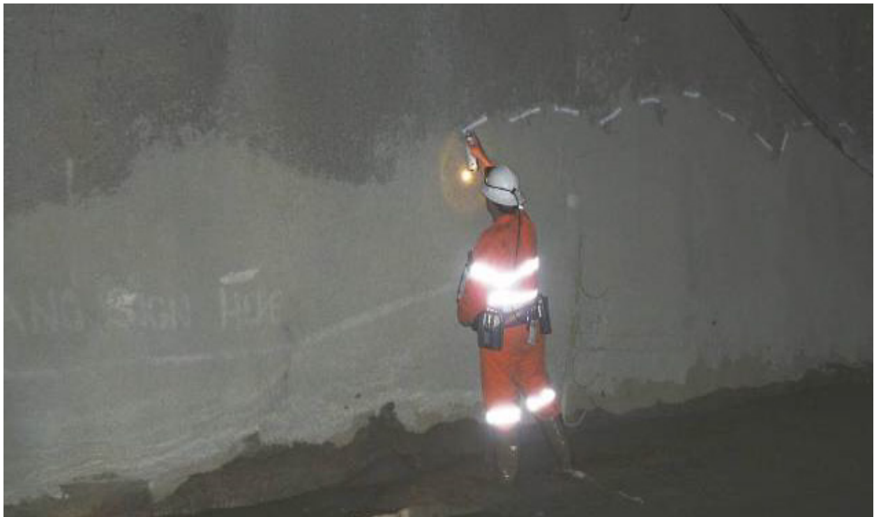
Photograph 1: Dried mud on the wall near VR5A shaft shows the height the material reached as it flowed to the base of the shaft.
