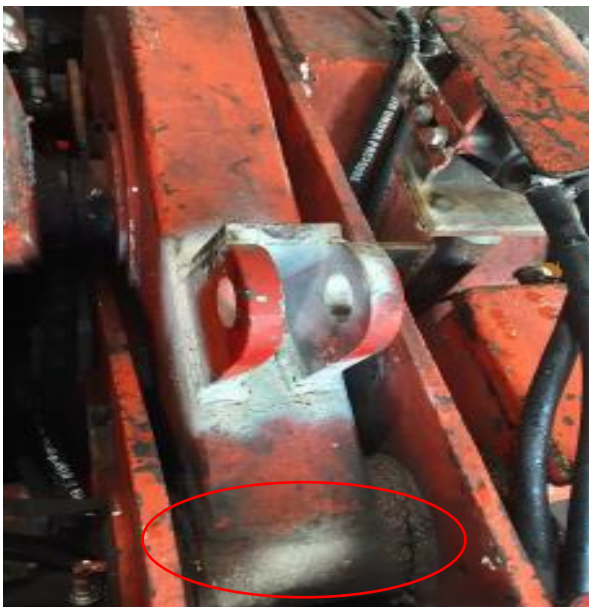
Figure 2: Area not accessible to NDT
